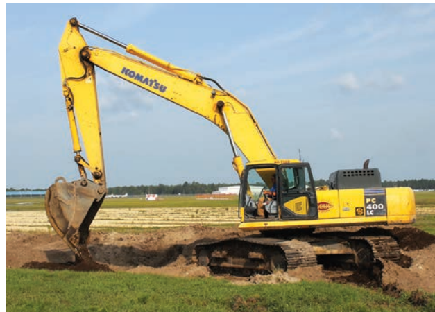
Gulf Coast Utility Contractors' Komatsu PC400 is at work at the Northwest Florida Beaches International Airport.
